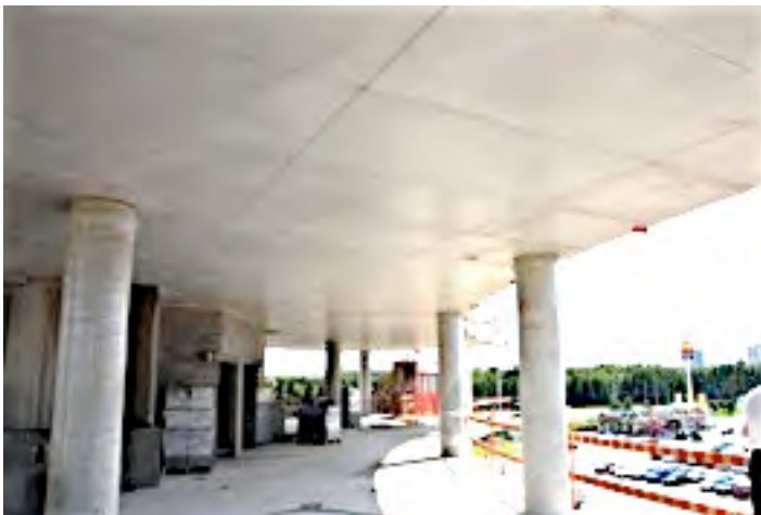
bottom surface with ultra fine tecture due to low viscosity of allmost self compacting concrete
