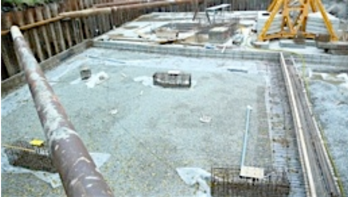
no additional reinforcement except in reentering corners and as connector between dayfields
